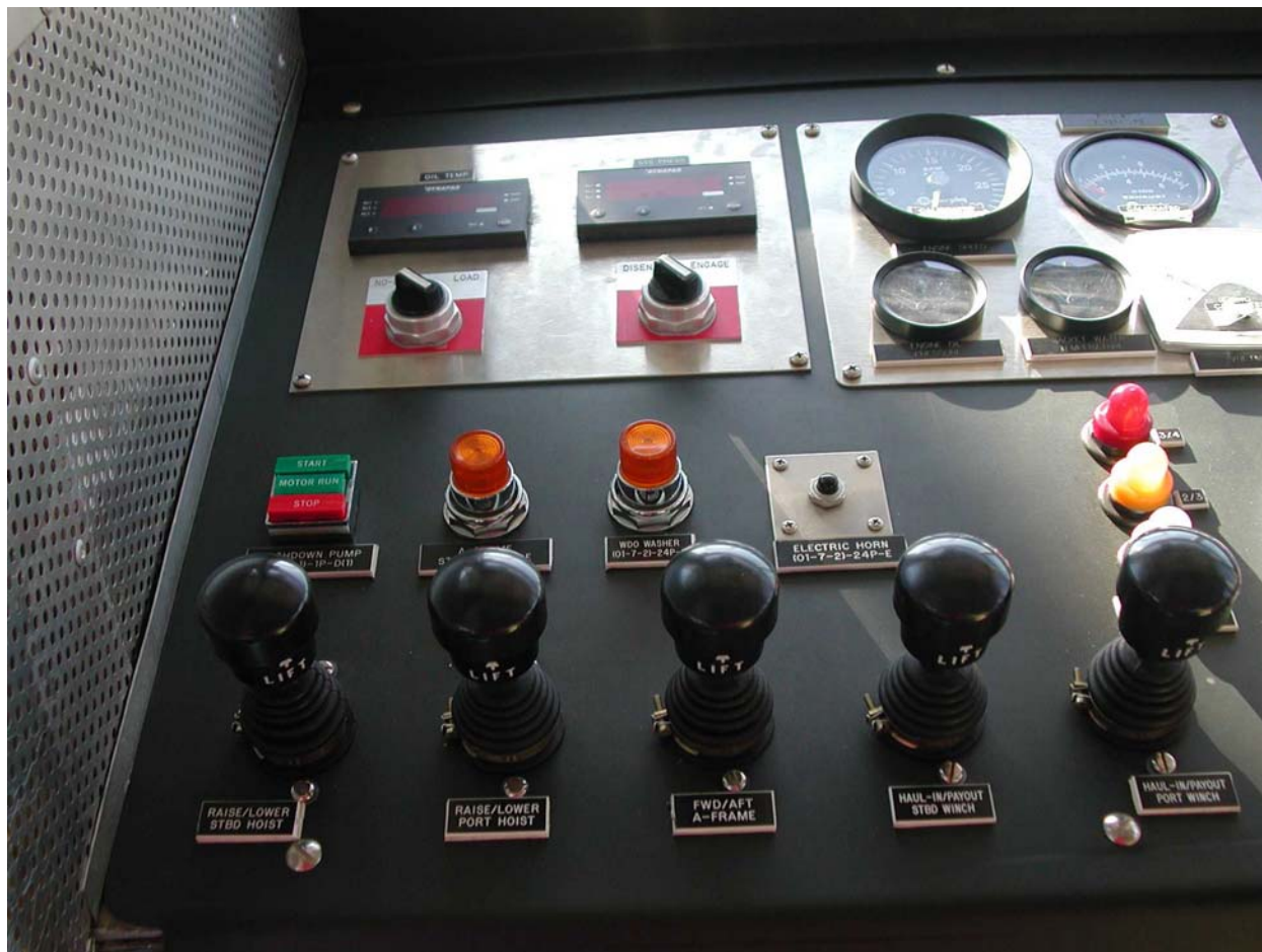
Figure 3-30 Aft Buoy Console Panel
