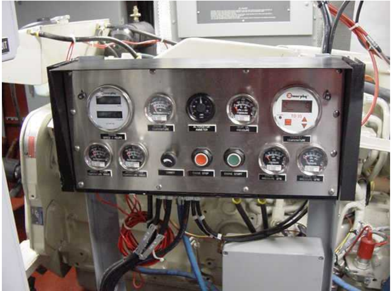
Figure 3-6 Engine Control and Gauge Panel - Machinery Space
