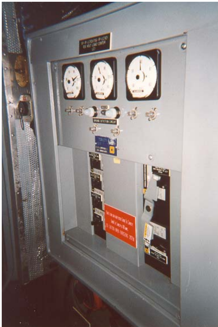
Figure 3-21 120-VAC Load Center (LC) 1
