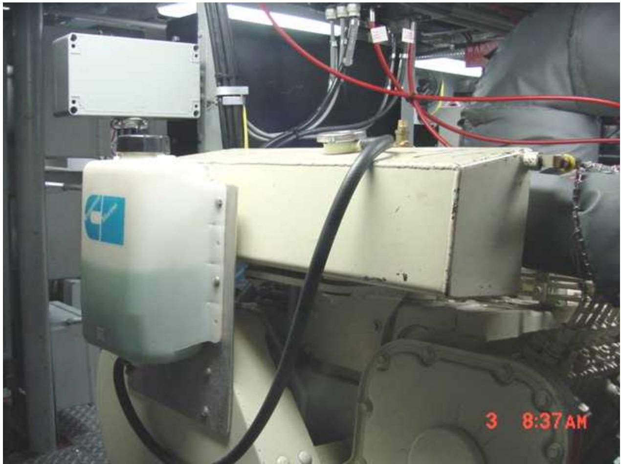
Figure 3-9 Main Diesel Engine Coolant Reservoir
