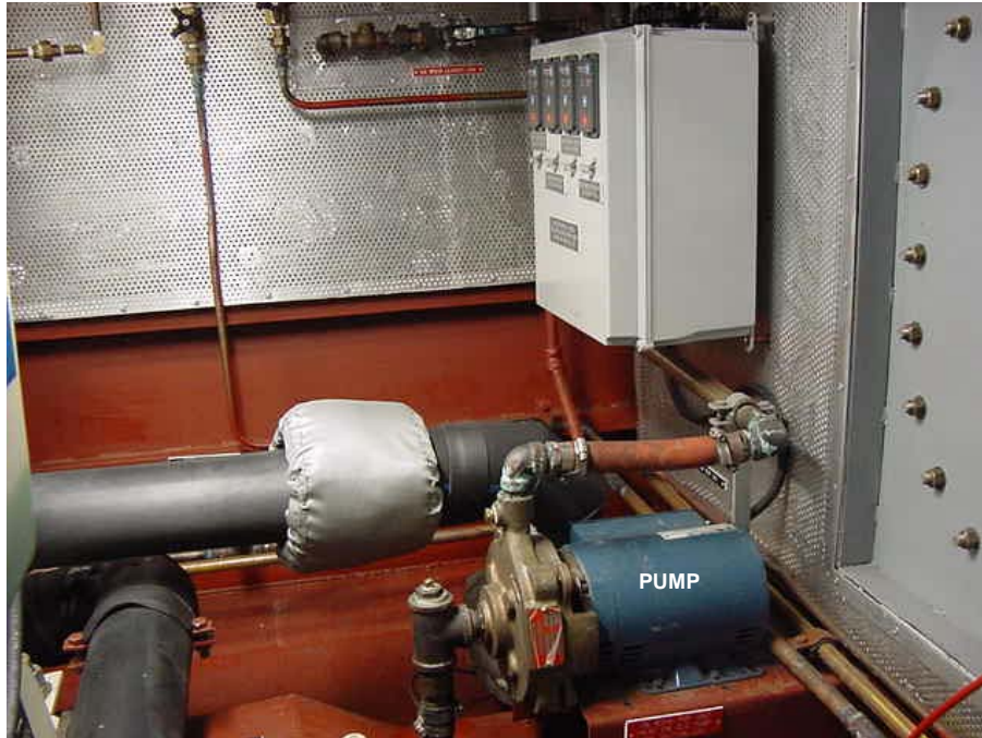
DECK WASHDOWN PUMP IN MACHINERY SPACE
