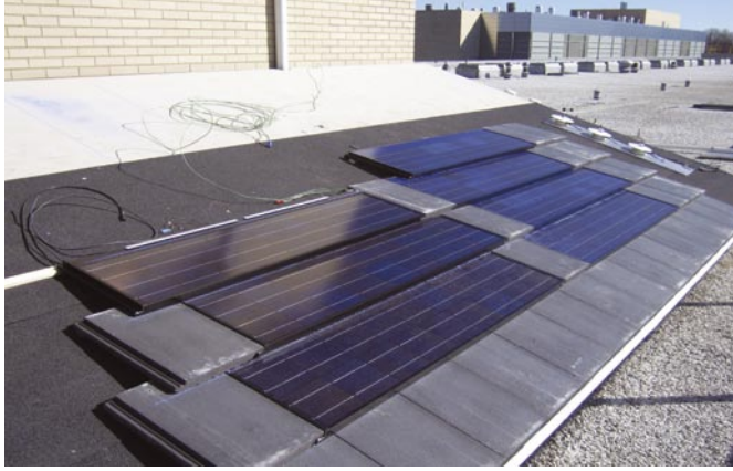
Residential Building Photovoltaic Panel.
