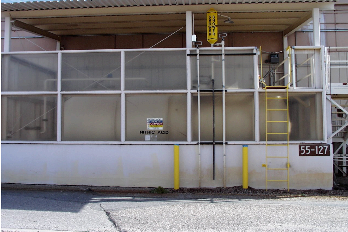
Figure 7-1. Nitric Acid Tank at LANL
