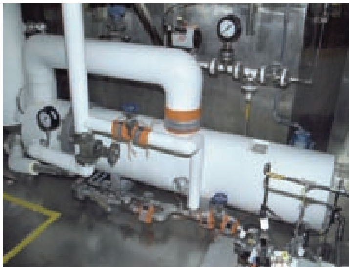
Figure 7-2. Nitric Acid Recycling System at LANL
