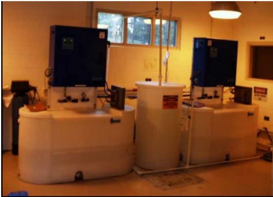
Fig. 7-1. MIOX system for treating sanitary waste.
