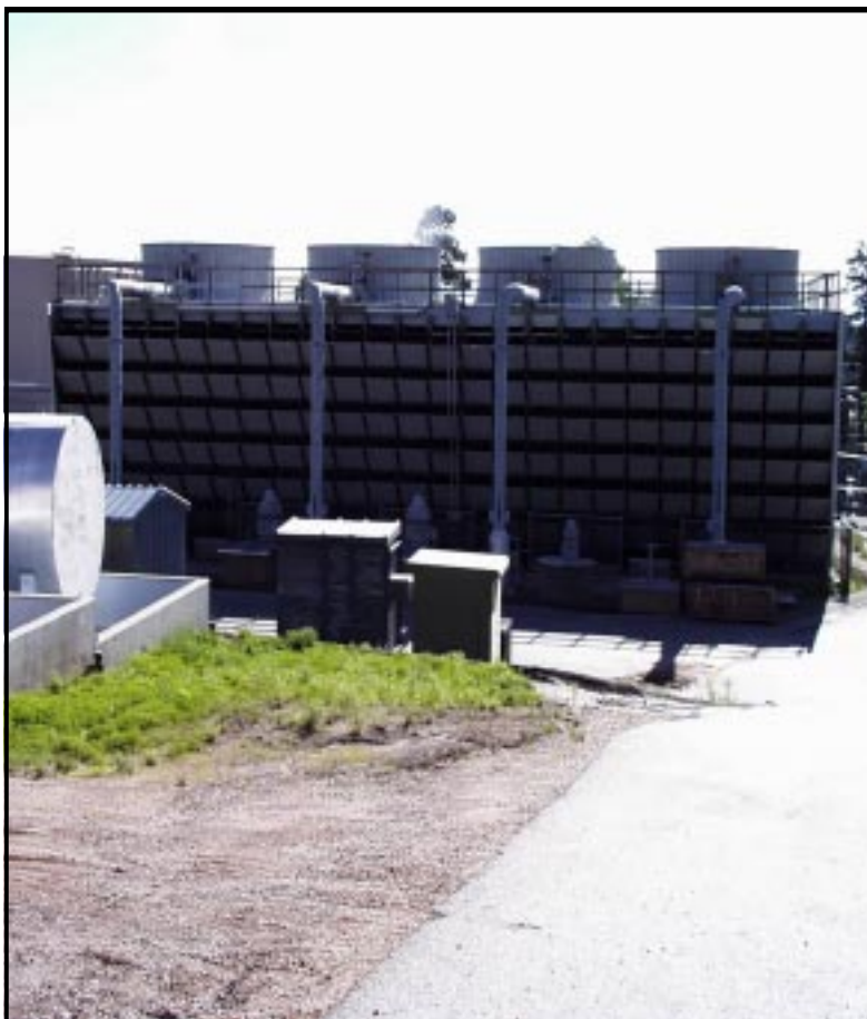
Fig. 7-2. Power plant cooling tower.
