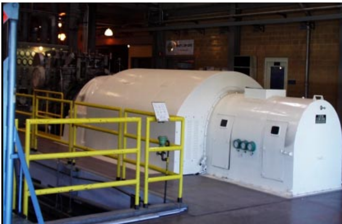
Fig. 6-1. One of several turbines at the Laboratory's power plant.
