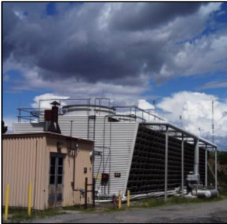
Fig. 7-3. Cooling tower at TA-53.
