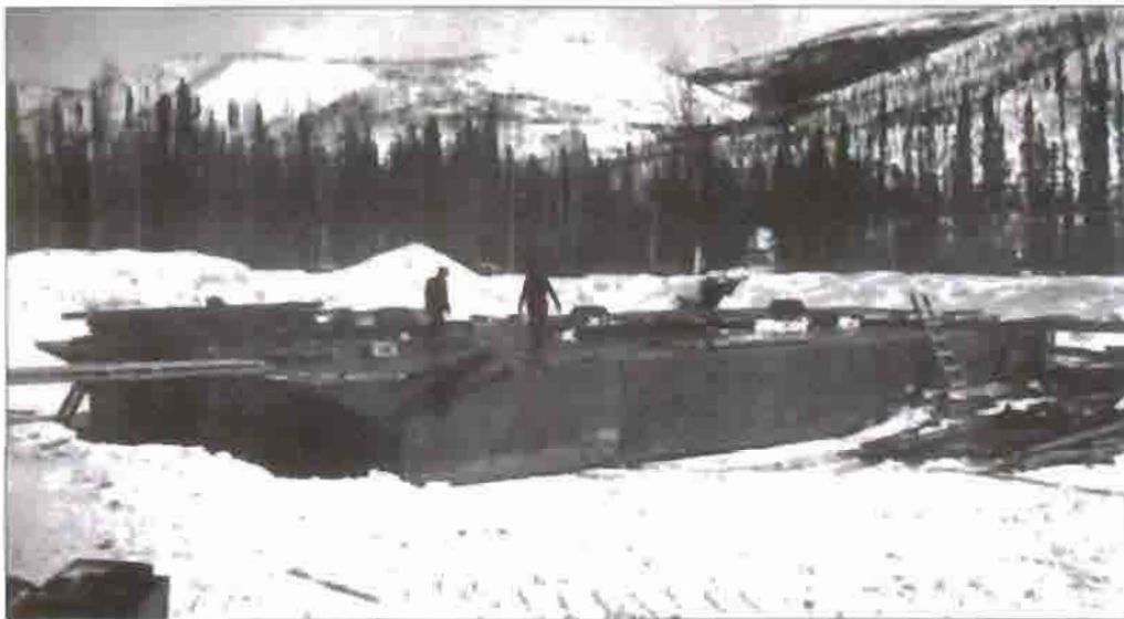
Metal "boxes" are assembled forming the pontoon hull are assembled on the frozen surface of the construction pond at Camp No. 1. NPS photo, Bill Lemm Collection.
