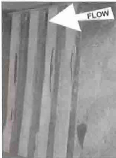
Figure 7: Riffles showing the wear occurring on the corner of the angle iron from the constant pounding of gravel and sand. The water flows in the direction indicated. NPS photo, Douglas Beckstead, July 2001.
