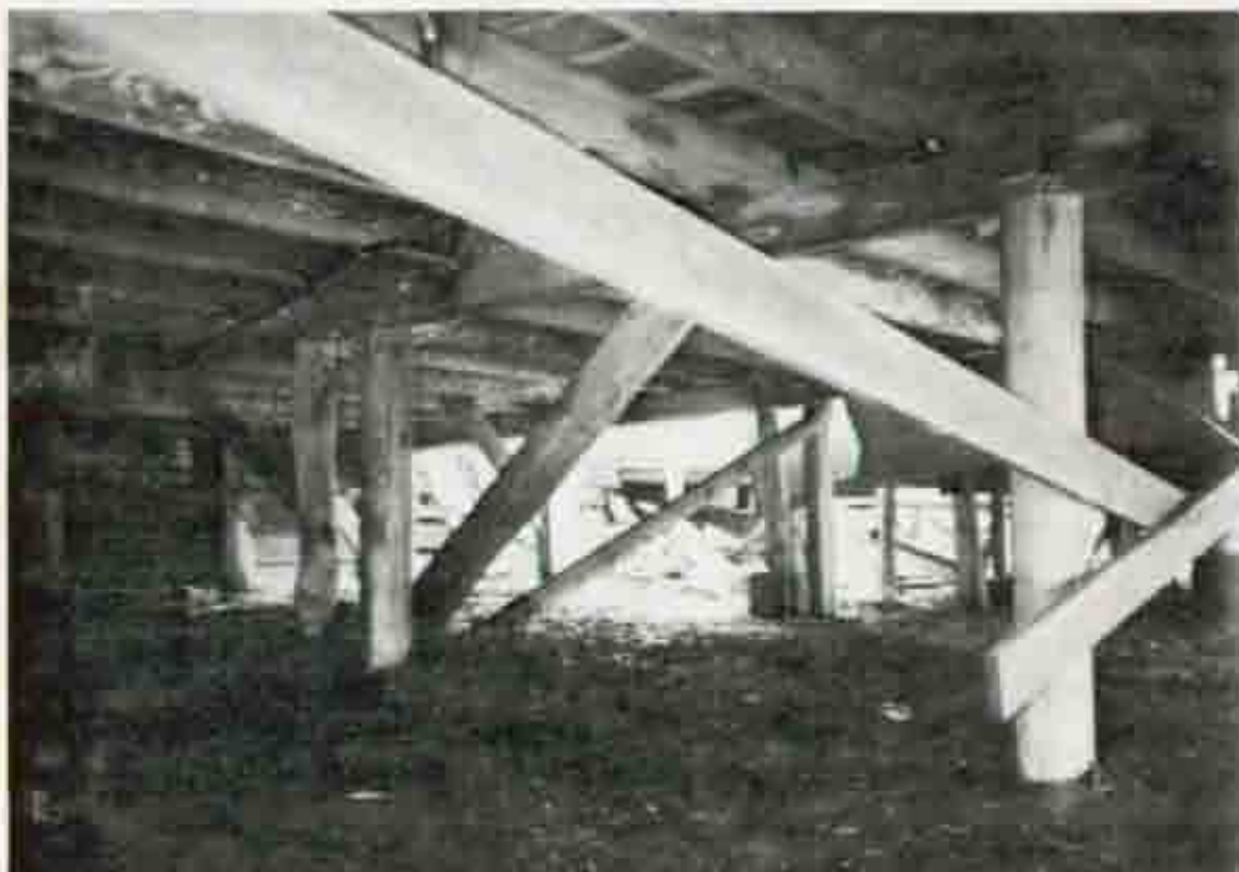
Figure 29 - Structure 17, Spiegel cabin, pilings and subfloor. Typical of all structures at Hamlet.
