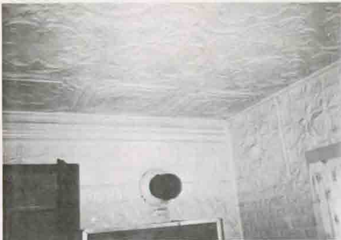
Figure 28 - Structure 17, Spiegel cabin, detail of pressed tin on kitchen walls and ceiling.
