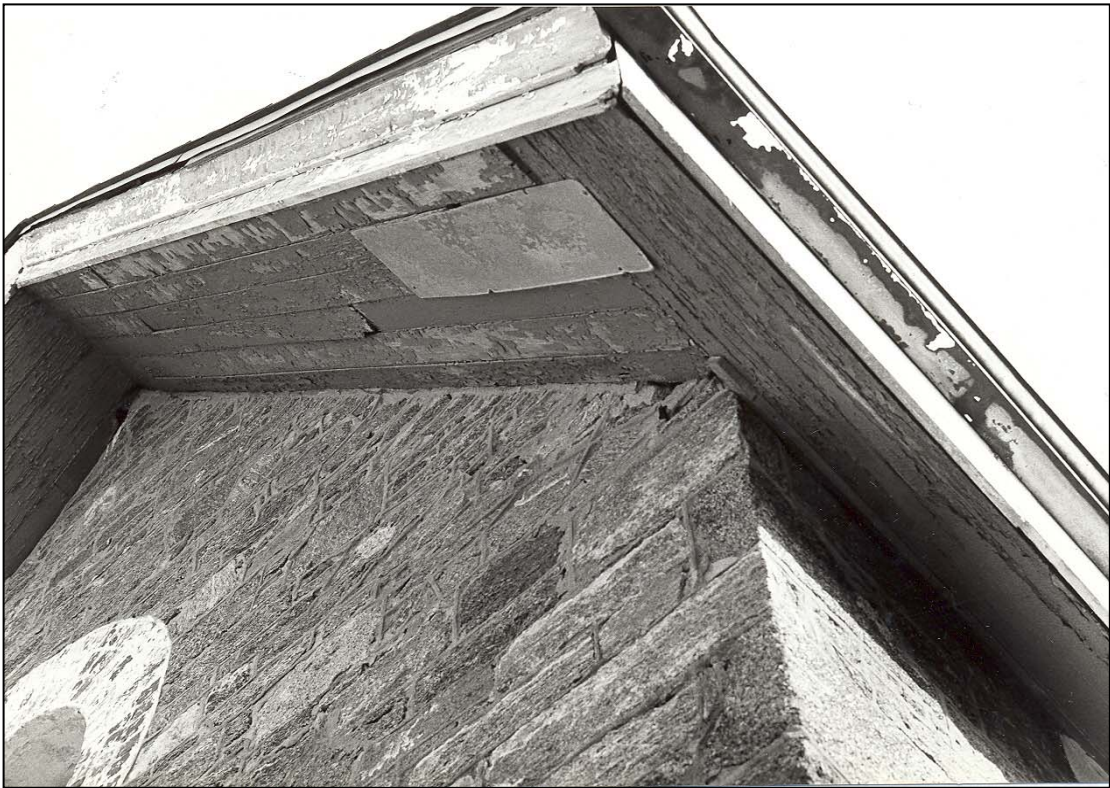
Figure 244. Dwelling exterior: north pavilion, soffit and fascia boards with crown molding and drip edge (1983).
