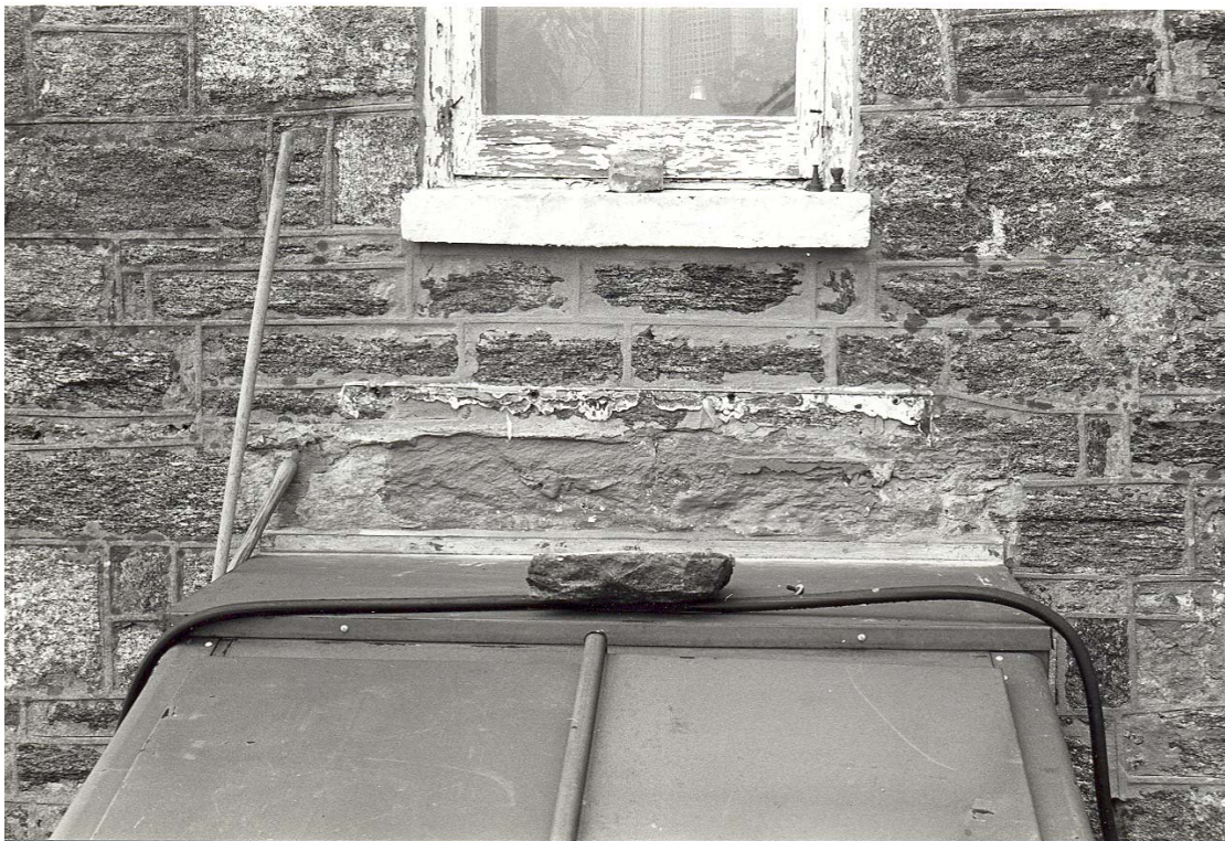
Figure 249. Dwelling exterior: north wall of east apartment, bulkhead and evidence for earlier bulkhead (1982).
