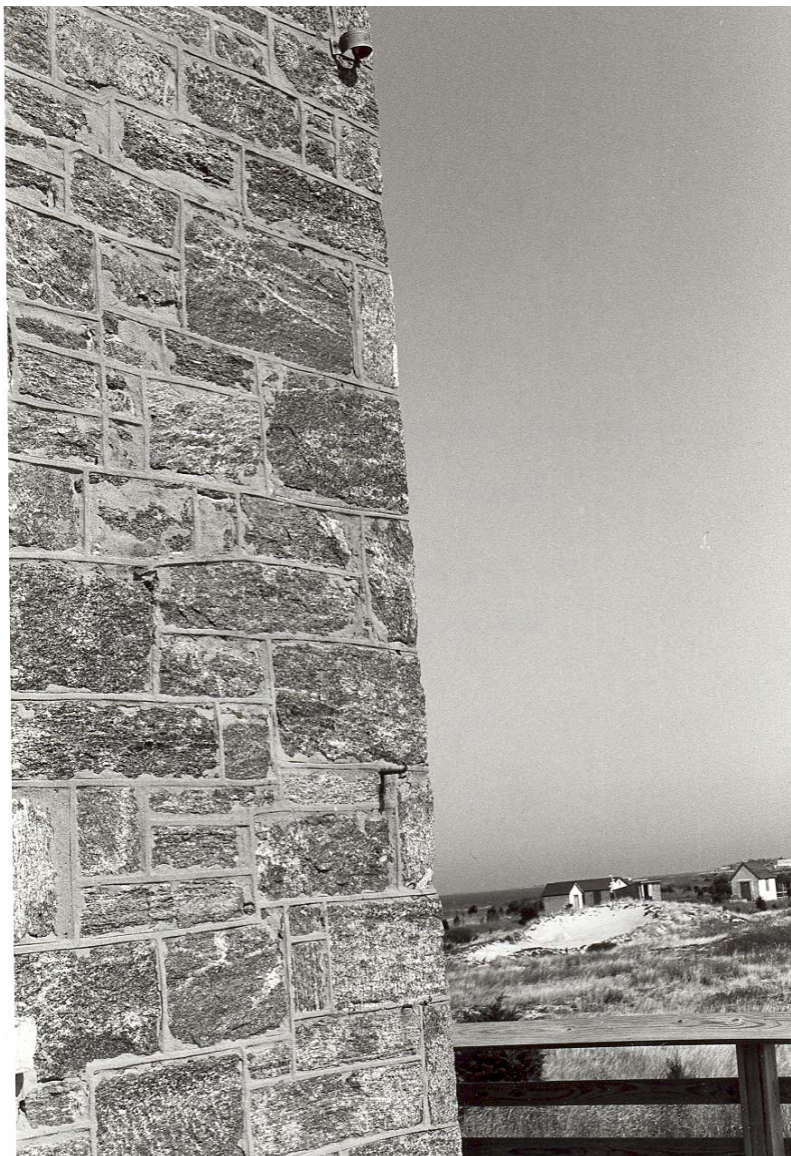
Figure 242. Dwelling exterior: east end of south wall, evidence for former downspout (1983).
