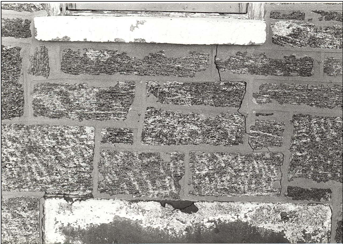
Figure 230. Dwelling exterior: south wall, masonry cracks (1983).
