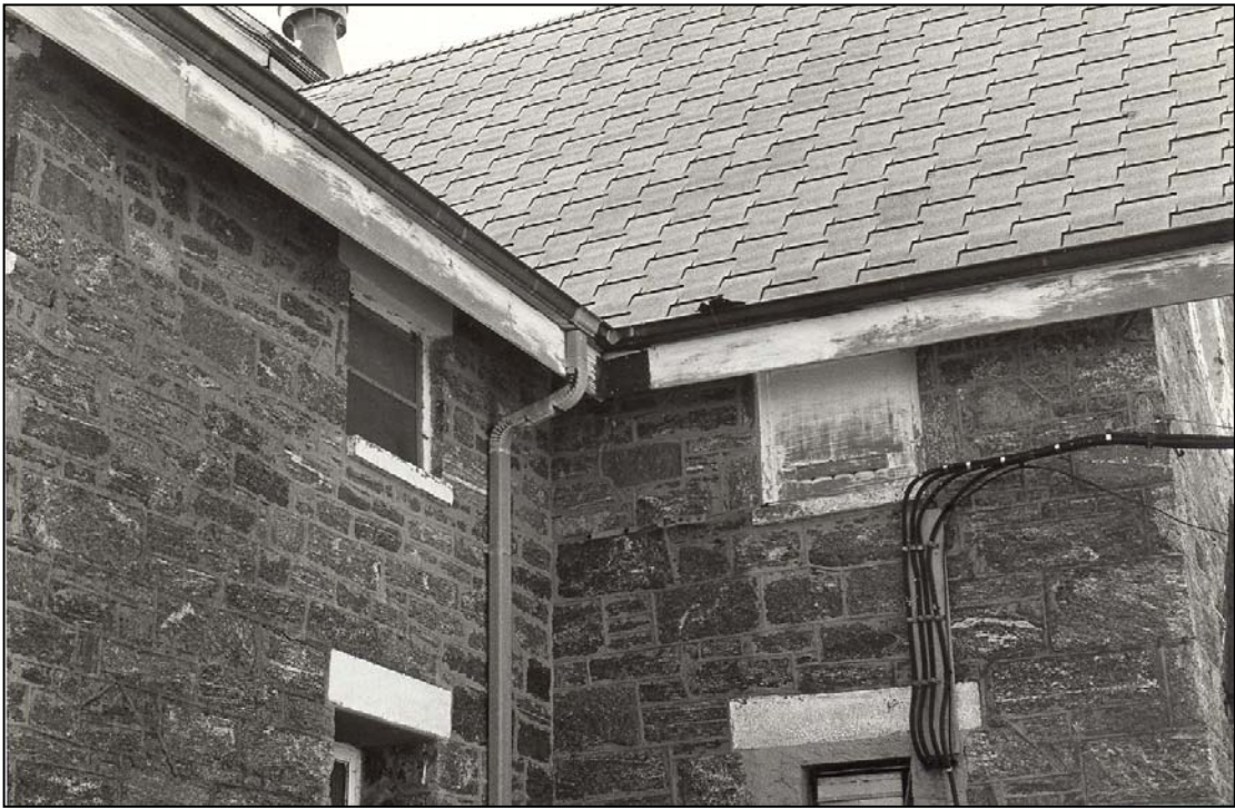
Figure 240. Dwelling exterior: Dwelling exterior: east junction of north wall and pavilion, with gutters, downspout, and fascia boards (1983).
