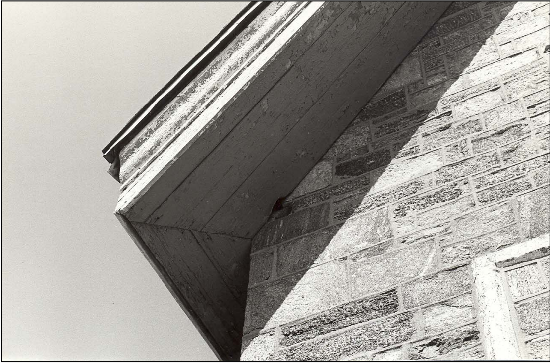
Figure 243. Dwelling exterior: Dwelling exterior: south pavilion, soffit and fascia boards with crown molding and drip edge (1983).
