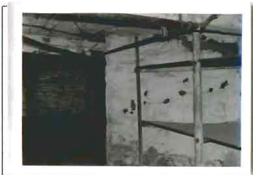
Photograph 9. D.R. Miller House. Cellar showing stone chimney pier (foreground) and puncheon insulation (top). Photo by Paula Reed. 6/91
