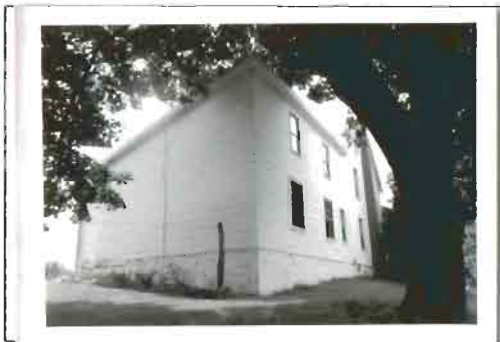
Photograph 4. D.R. Miller House, southeast view with rear addition. Photo by Paula Reed. 6/91
