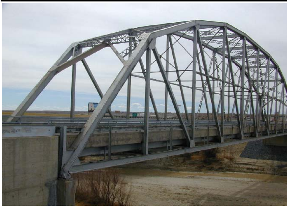
Rio Puerco Bridge, west of Albuquerque, completed in 1933. An example of the property type Bridges, this is a splendid Parker Camelback Through-Truss bridge. Photo: Michael Cassity, 2004.
