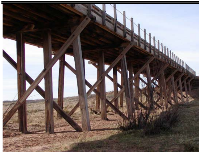
Timber Bridge west of Endee, New Mexico. Photo: Credit, National Park Service, Route 66 Corridor Preservation Program, Santa Fe, New Mexico, 2003.
