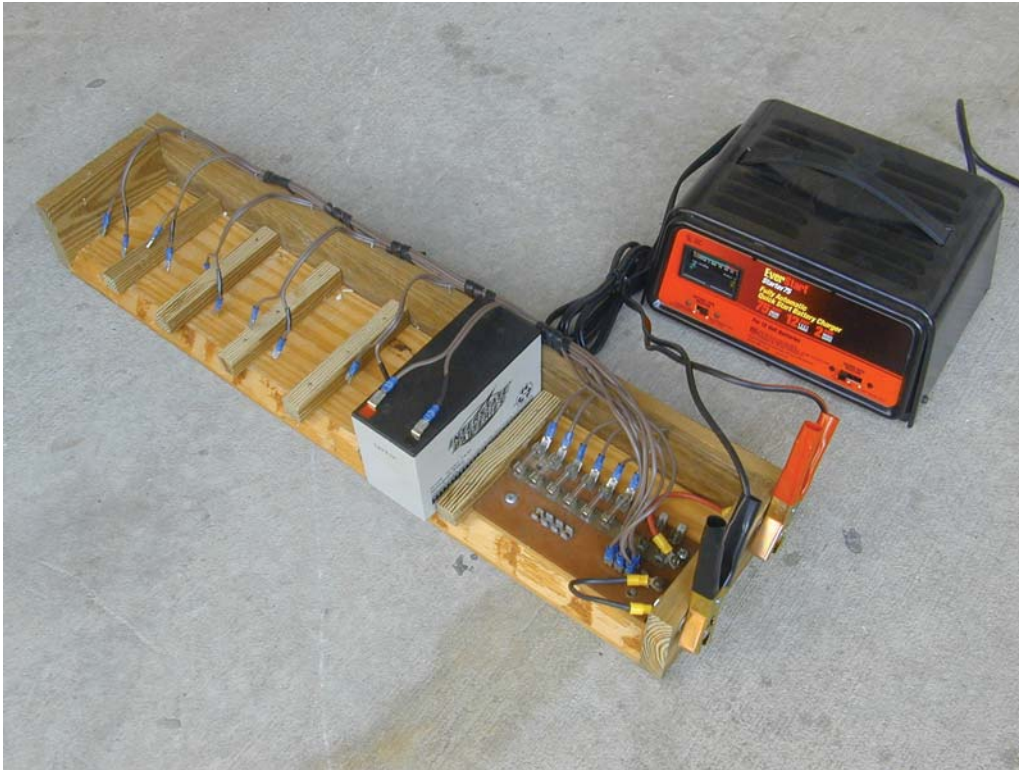
Figure 5. Example of a six battery bank charger. Each battery is individually fused to prevent catastrophic failure should an accidental short occur.
