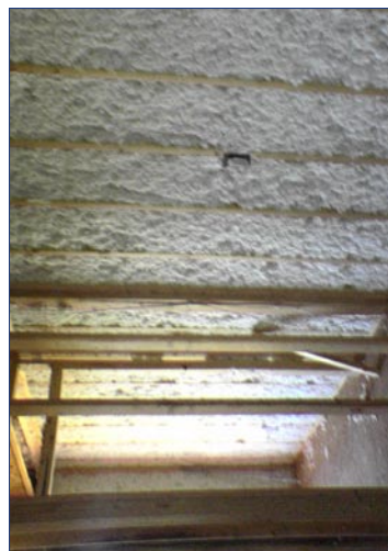
Walls are 2x4 studs insulated with blown-in fiberglass to R-15 plus two inches of extruded polystyrene (R-10).
