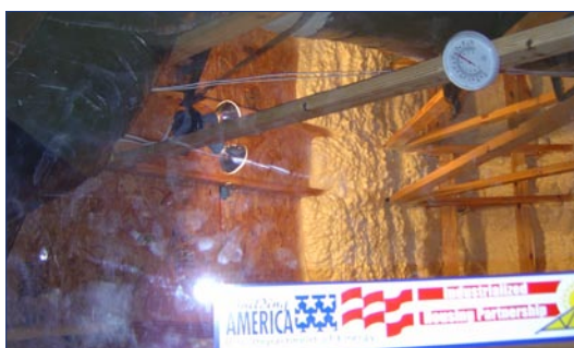
Shoppers love to peer into the attic through this viewing window in a Building America model house by Cambridge Homes. Shoppers can see the special insulation, and the thermometer tells them how cool the attic stays.
