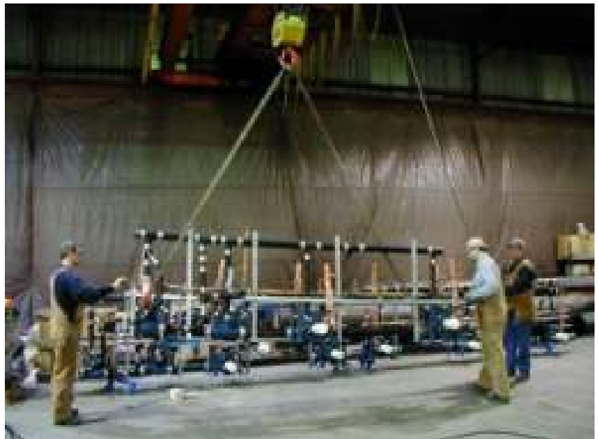
Figure 26 Overhead crane eliminates hazards, saves time and effort and protects finished product
