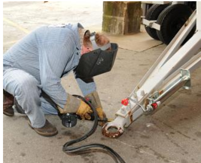
Figure 36 Before: Welder's neck and back are in an awkward posture while he kneels on a hard surface
