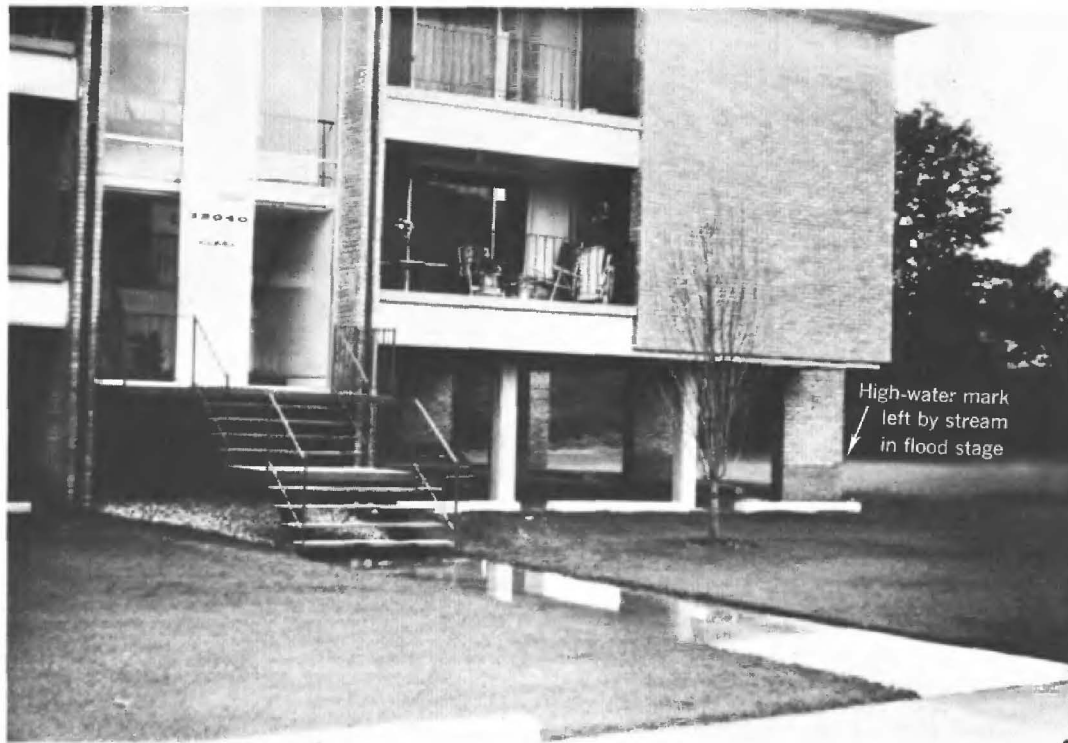
Structure built on stilts reduces possibility of damage by flood water. Notice high-water marks left by stream in flood stage on building supports in right center of photograph. FIG. 89
