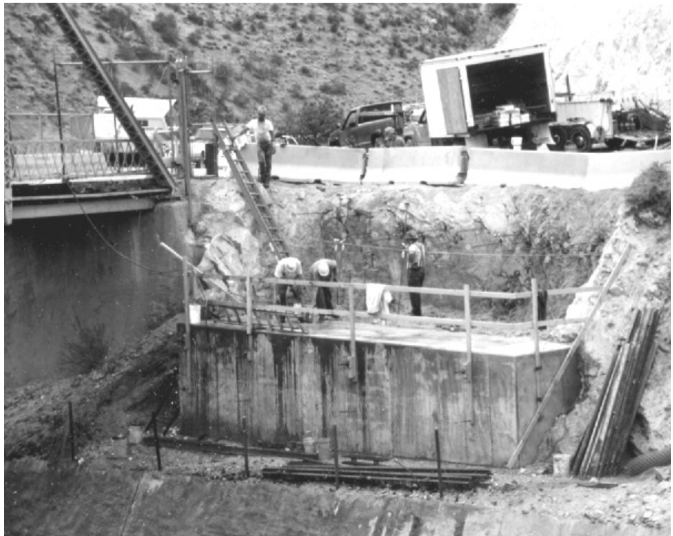
Construction crews are on location at Arrowrock Dam, building a new access bridge and preparing to replace Ensign valves in the nearly 90-year-old structure.
