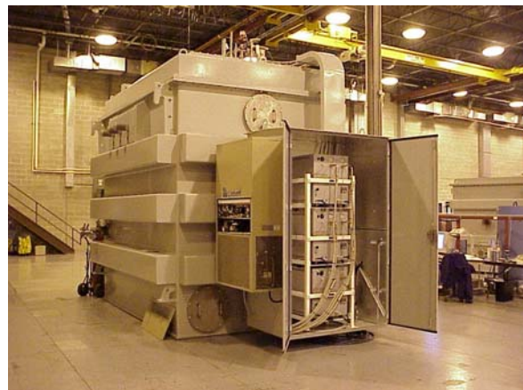
Fig. 2.31. Completed transformer showing compressor cabinet.
