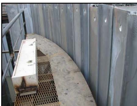
6. Template with a full set of sheet pile. Template curvature matches design curvature of cell face.
