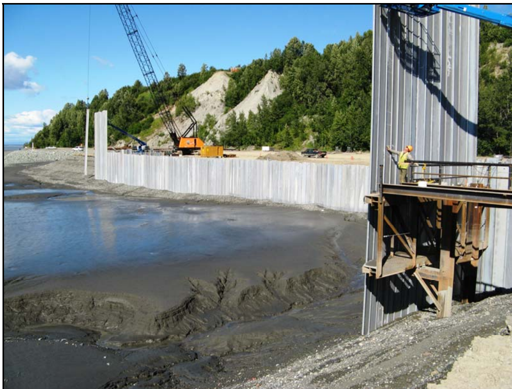
Figure 4(b). Barge Berth Construction 2008 APU Observation Station visible (orange) on Cairn Point Bluff
