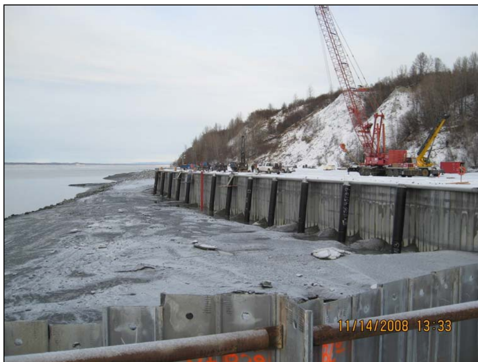
Figure 11(a). Sheet pile cells, barge berth construction site, low tide. View facing north.
