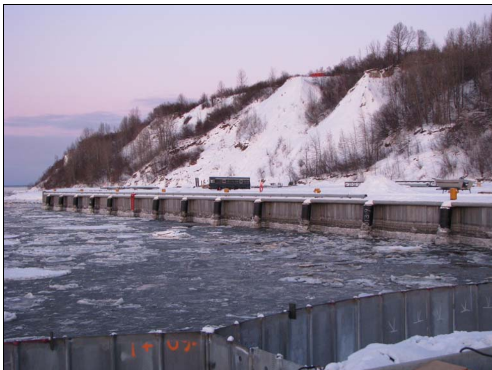
Figure 11(b). Sheet pile cells, barge berth construction site, high tide. Dec. 11, 2008. View facing north. APU Observation Station on bluff in background.
