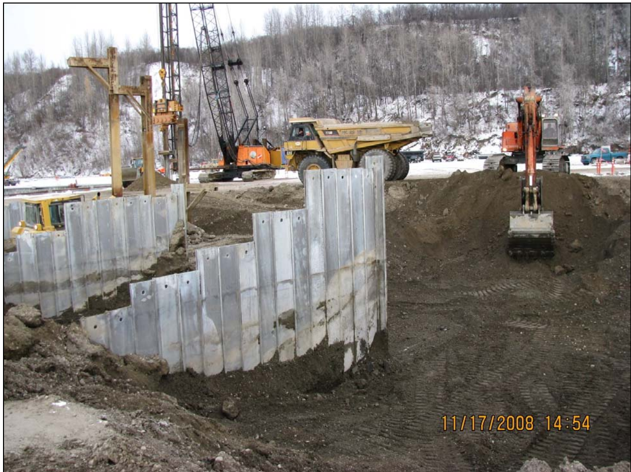
Figure 10. Out-of-water construction activities at barge berth site: constructing the tail walls of sheet-pile cells. View facing east.
