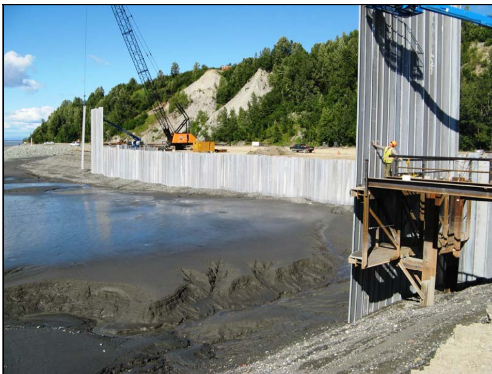
Figure 4(b). Barge Berth Construction 2008 APU Observation Station visible (orange) on Cairn Point Bluff
