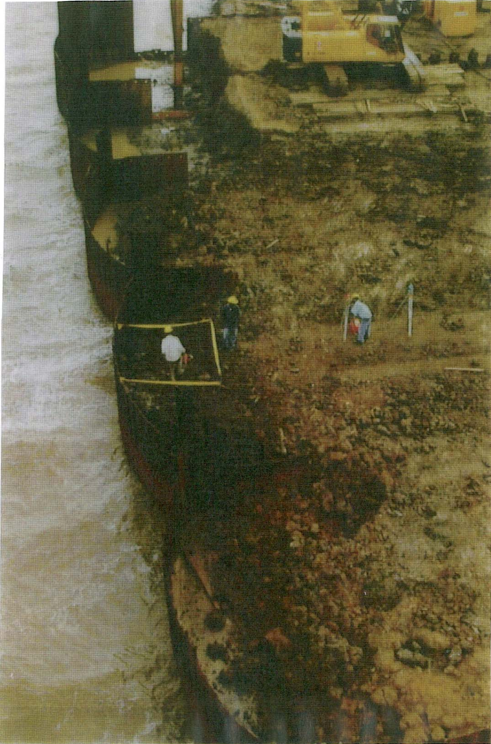
Figure 7 Fill Material Being Placed During Construction of an Open Cell Sheet Pile Dock
