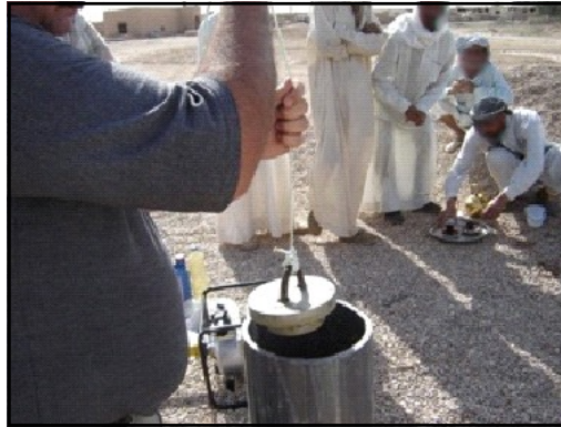
Workers perform an alignment test on a newly drilled well in a rural community in central Iraq; the well was drilled as part of USAID's rural water initiative
