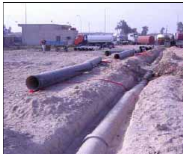
Refurbishment of a water treatment plant in Karbala will supply safe water and improve sanitation.
