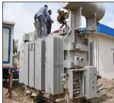
Iraq workers are installing 24 power substations in Baghdad, improving electricity reliability for 2 million Iraqis.
