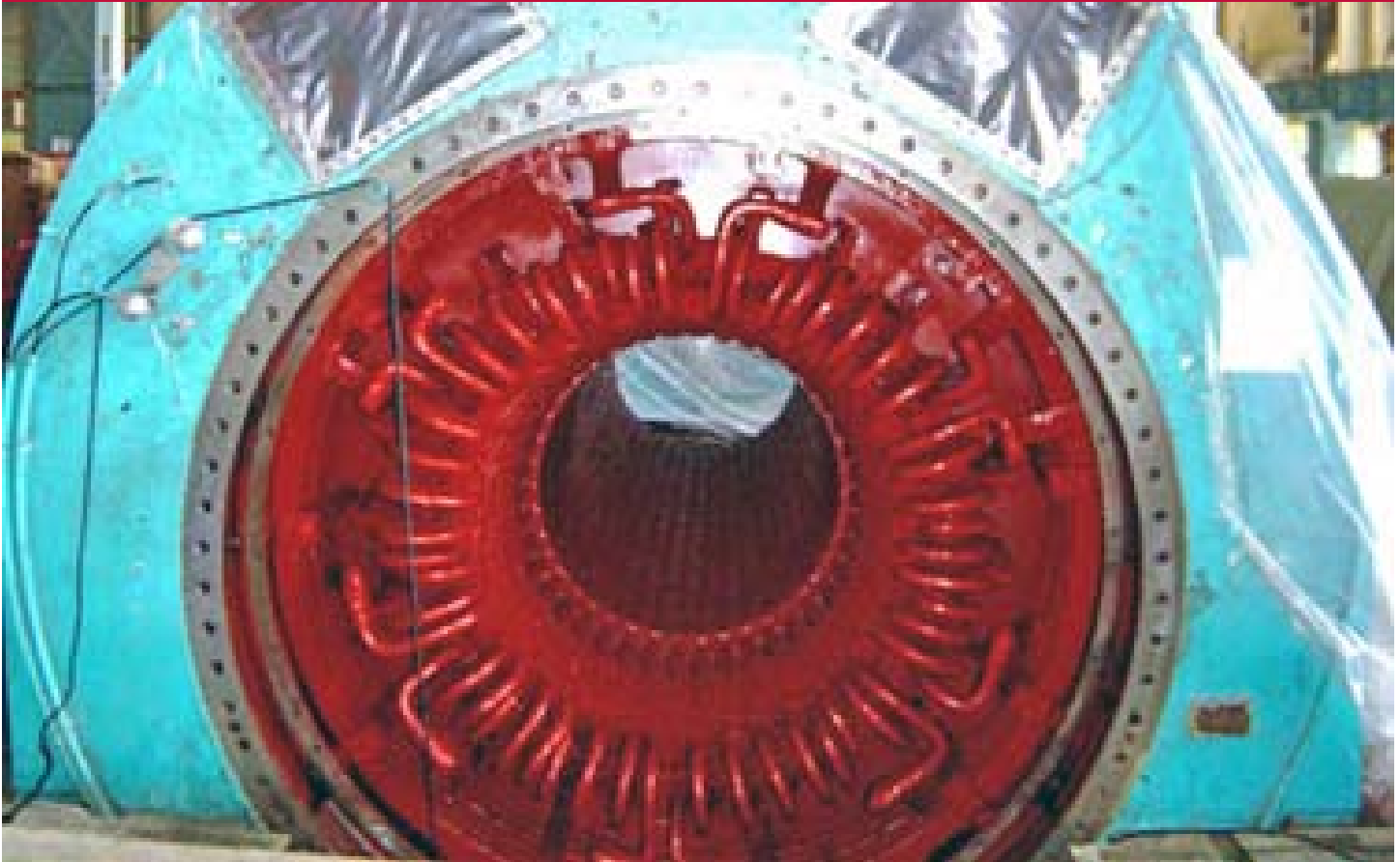
A new generator ready for testing and rotor installation at a power generation facility in southern Baghdad.
