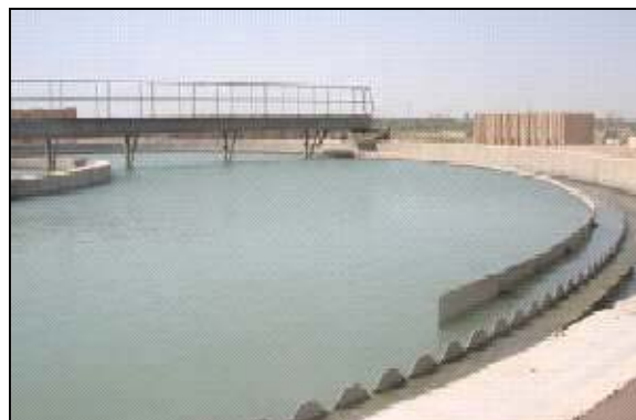
The Najaf Water Treatment Plant supplies potable water to the majority of the 563,000 city residents
