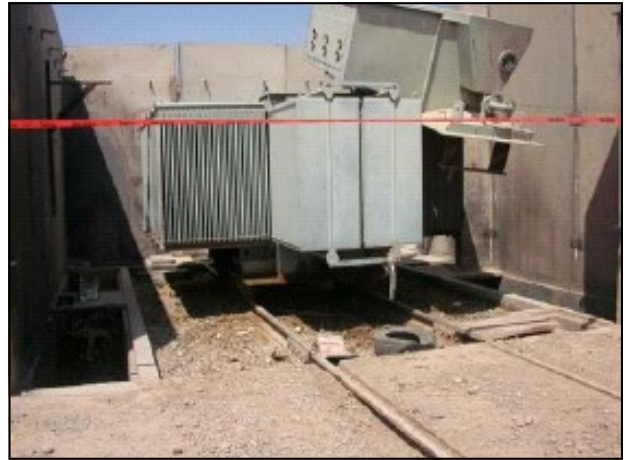
A new transformer for a Baghdad substation.
