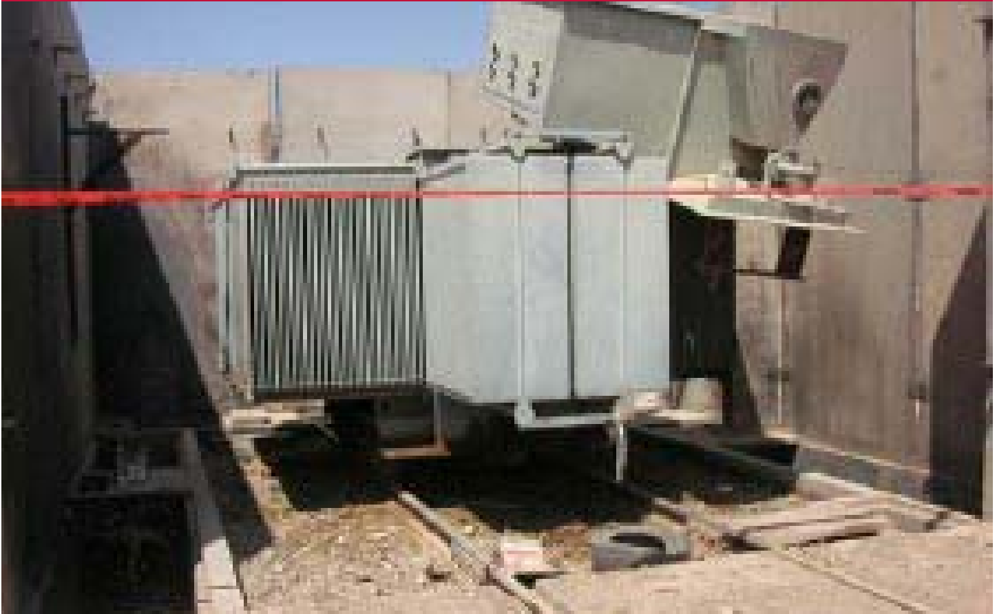
One of four temporary mobile substations that will substitute for Baghdad substations under repair by USAID
