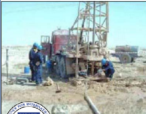
Workers prepare to drill a new well as part of USAID's rural water initiative.
