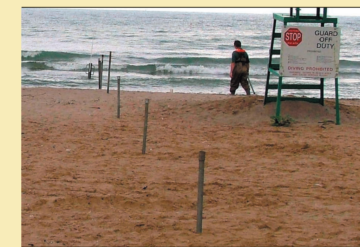
Figure 4. Locations of temporary piezometers installed in the lake and at 0, 3, 6, 9, 20, 40, 60, 80, and 100 ft inland from the water's edge in July 2004.
