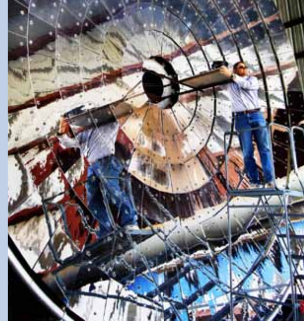
Project staff member adjusts solar tracking heliostat on a solar thermal collecting dish.
