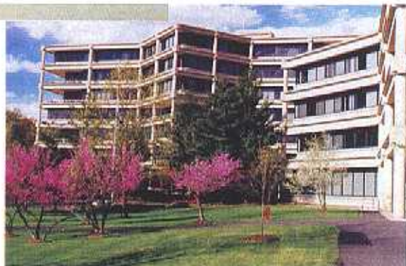
The Powell Building in Reston, Virginia, was studied to verify the effects of pollution on its poured concrete columns. The study included visual and tactile examination, wash-down experiments, and a quantitative examination of coarse pores (p. 64). Courtesy of the U.S. Geological Survey.
