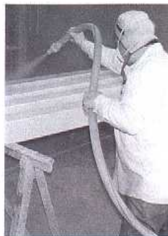
Surface preparation is key to a successful duplex system when painting over hot-dip galvanized steel (p. 44). Here, a worker uses aluminum/magnesium silicate to sweep-blast galvanized steel before a coating is applied. Courtesy of the American Galvanizers Association.
