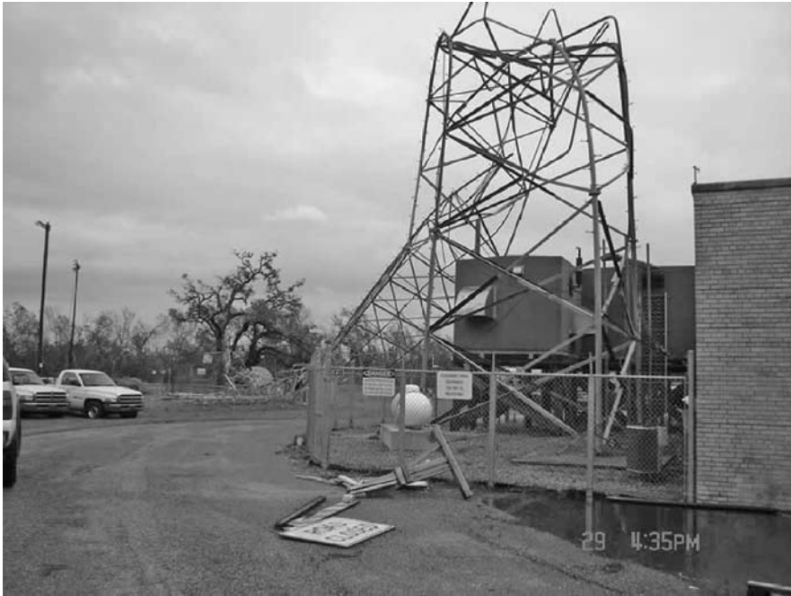
Figure 16-9: Plaquemines Parish (Louisiana) Radio Tower – August 29, 2005
