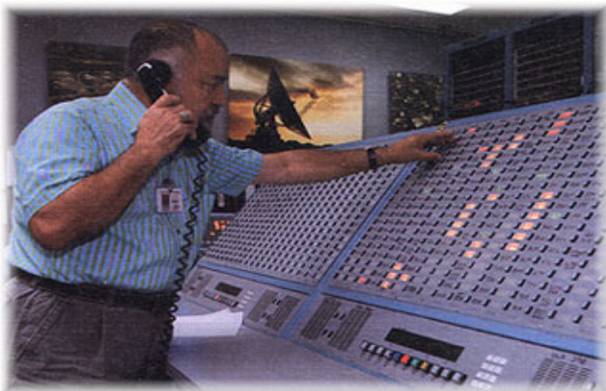
Voice Switching System (VSS)
