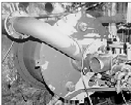
Southern Company Services' Demonstration of Advanced Combustion Techniques for a Wall-Fired Boiler, Low-NO x burner mounted into its boiler penetration with igniter installed.
