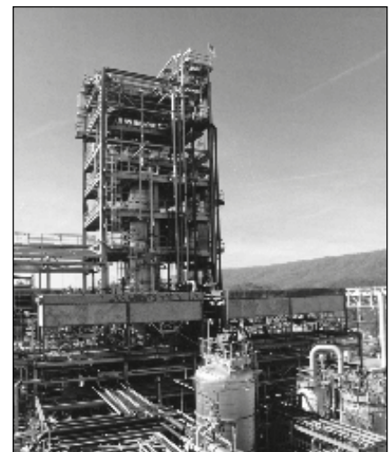
This project demonstrates at a commercial scale the LPMEOH™ process to produce methanol from coal-derived synthesis gas.
