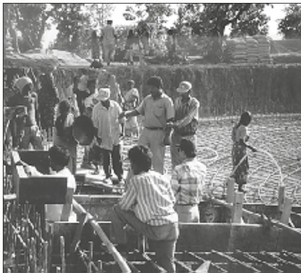
Workers prepare foundation at the Bilaspur Coal Washery Project in Madhya Pradesh, India.
