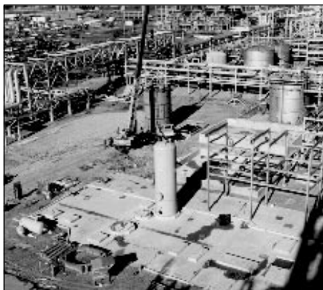
The LPMEOH™ project will start operations this fall and will demonstrate the coproduction of methanol and electric power.
