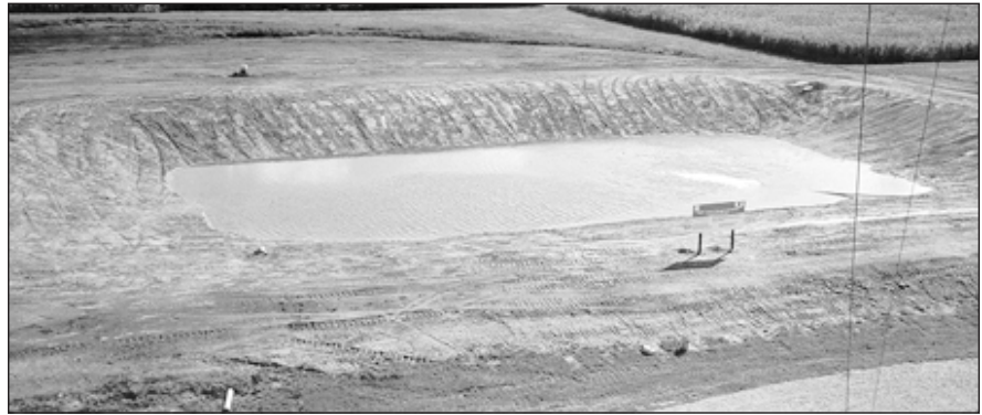
Figure 1: Animal waste storage lagoon constructed with low-permeability FGD/fly ash liner (photo courtesy of Ohio State University)
