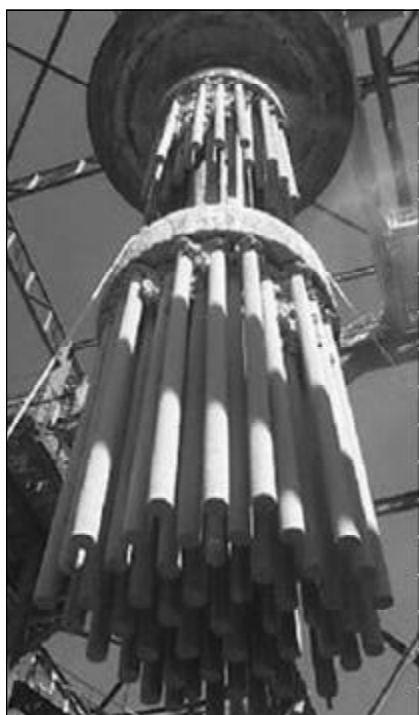
Candles from the inside of the Siemens-Westinghouse candle filter vessel
