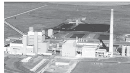
The Holcomb Station in Finney County, Kansas is a 360-MW wall-fired boiler burning Powder River Basin coal
