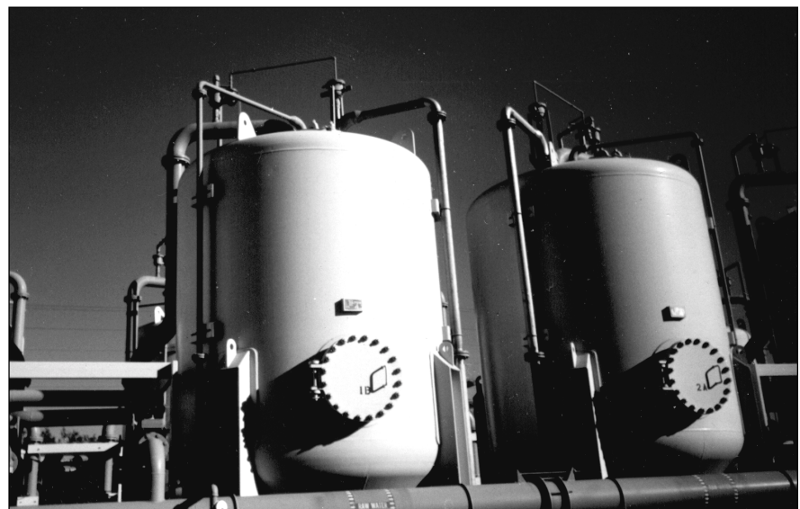
Activated carbon treatment tanks, in Redlands, California, being tailored for the removal of perchlorate from water.
