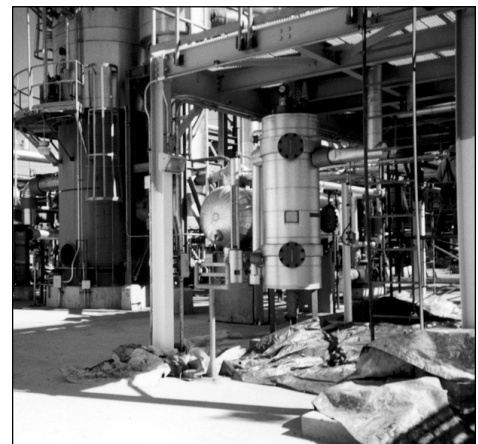
State-of-the-art CO 2 scrubbing facility is located at coal-fired Warrior Run Power Plant in Cumberland, Maryland.
