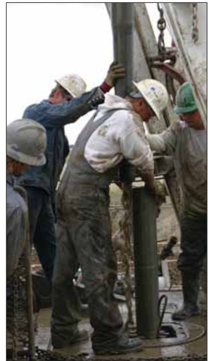
Workers drill a CO 2 injection well in North Dakota as part of a PCOR project
