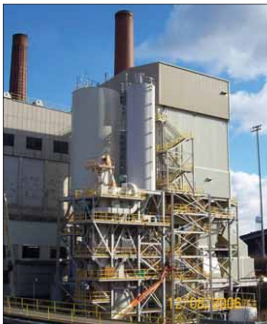
View of Greenidge scrubber and baghouse
