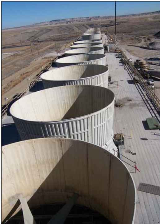
View from top of Air2Air™ test cell
