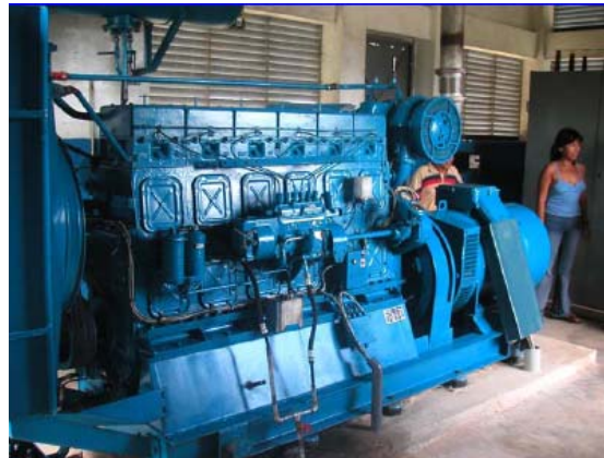
Fig. 6. 100-kW diesel generator.
