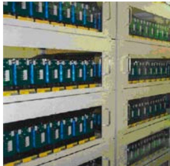
Fig. 23. Large electrochemical capacitor storage system that provides short-time uninterruptible power. (Photo courtesy of Nippon Chemi-Con)
