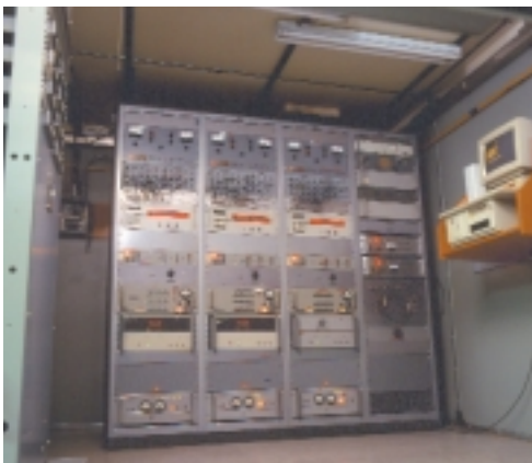
Figure 3.6. WWV Control Room
