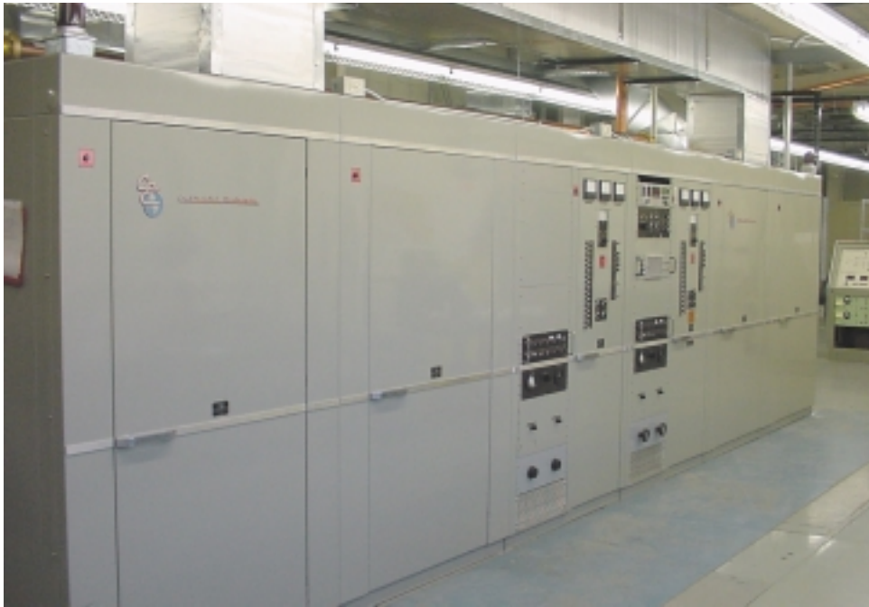
Figure 2.4. A WWVB Transmitter
