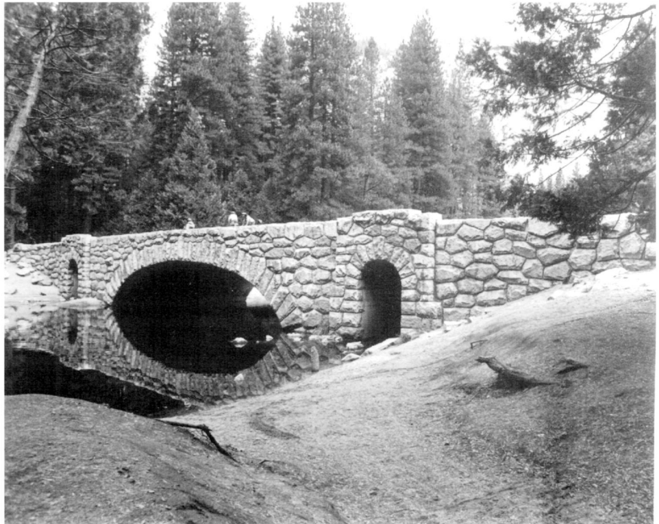
View showing the east facade of the Stoneman Bridge, Yosemite National Park, Mariposa County, California, designed and built by the National Park Service in 1933. The bridge is reinforced concrete faced with rough boulders of native granite to give it a rustic appearance. The photograph shows the exterior material very clearly and also shows significant features—the equestrian tunnels—and how they are built out from the face of the wing walls for decorative emphasis. (National Park Service. Dean Shenk, 1976)
