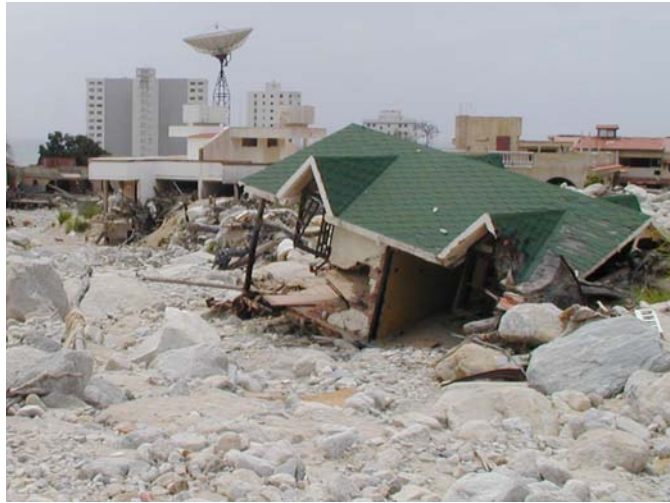
This house was carried and rotated by debris flows in Caraballeda, Vargas, Venezuela, 1999.
