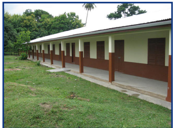
MCC funds the construction and rehabilitation of schools in 30 districts, providing students and teachers with safe structures, potable water, latrines, and furniture. In collaboration, USAID is identifying, training, and employing members of the community to teach in these MCC-funded schools.
