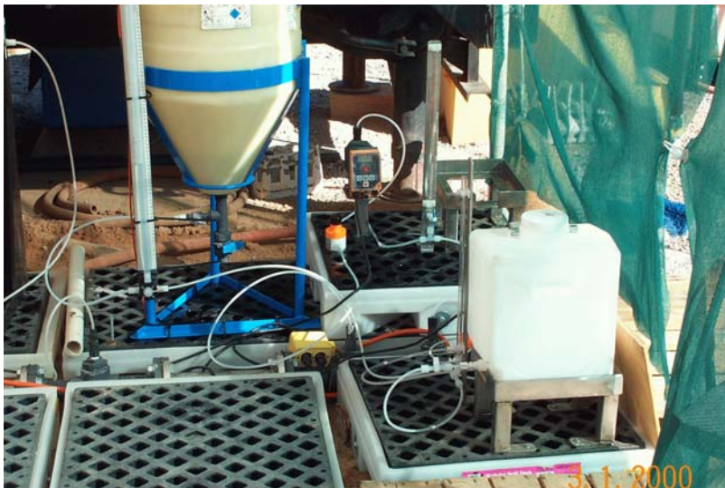
Figure 8.—Acid feed system (sulfuric acid), with spill pallet, 17-gallon supply tank, calibration cylinder, and back pressure valve.
