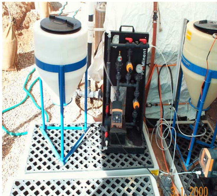
Figure 10.—Ammonia feed system (ammonia sulfate), with spill pallet, 17-gallon supply tank, calibration cylinder, bypass relief line, pulsation dampener, and back pressure valve.
