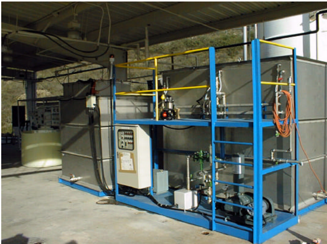
Mitsubishi MBR Pilot Unit
