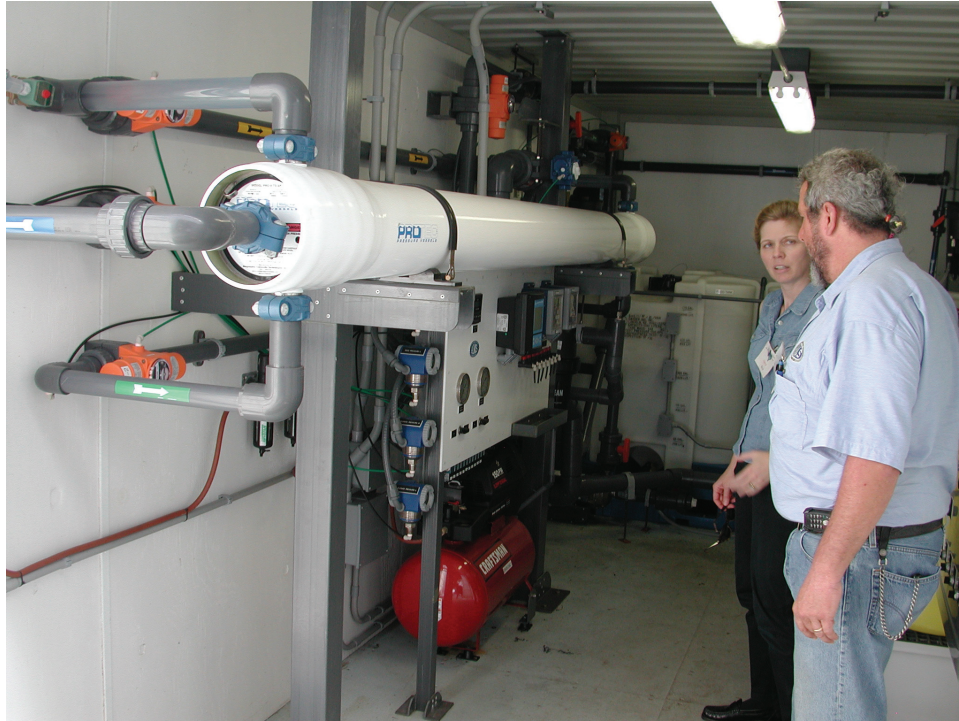
Figure 5.3. Membrane filtration X-Flow pilot unit provided by Norit Americas.
