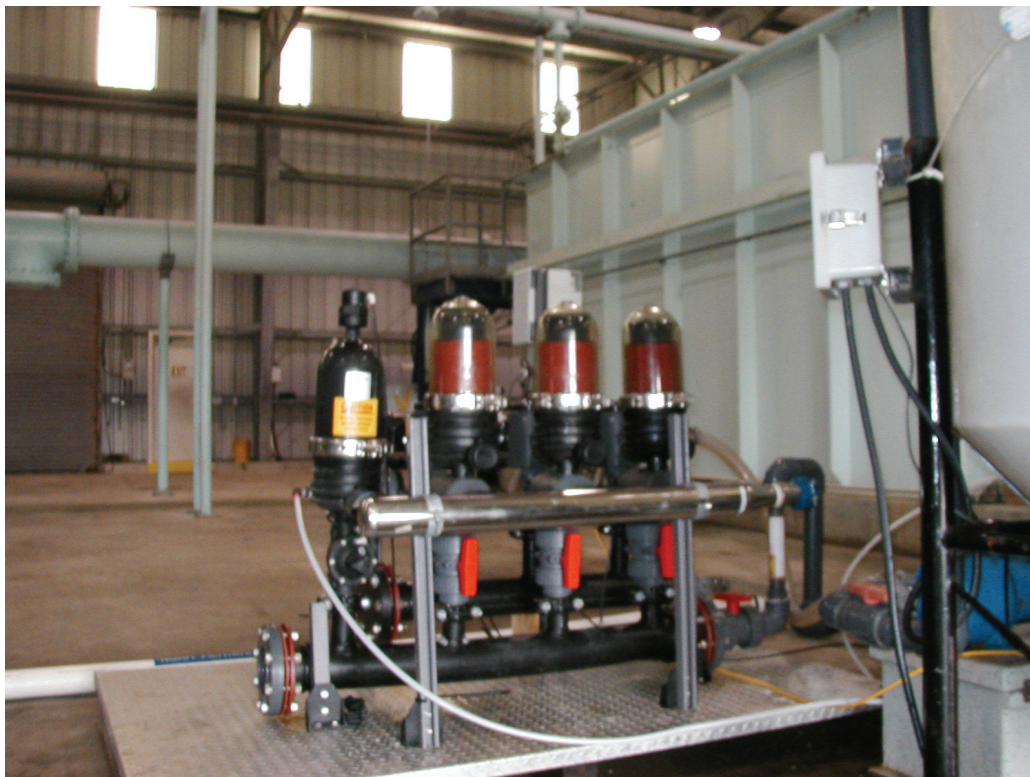
Figure 5.2. Installed disc pre-filtration technology.
