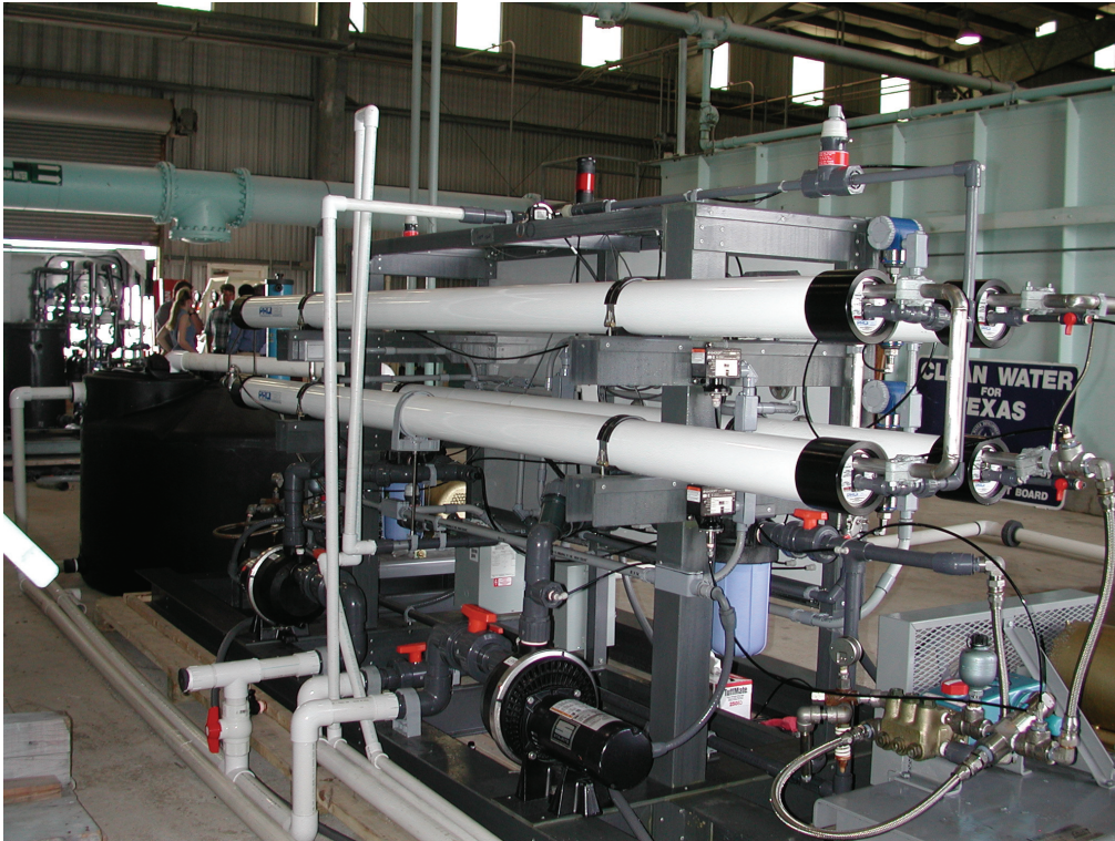
Figure 5.7. Back view of RO pilot system.
