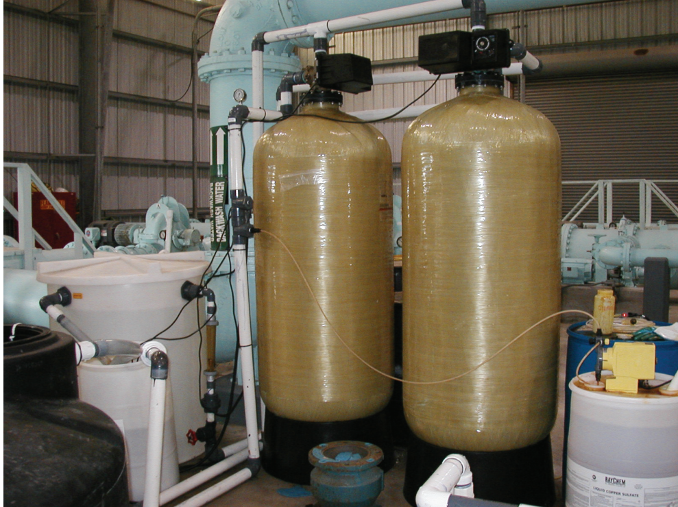
Figure 5.5. Conventional media filtration pilot unit.
