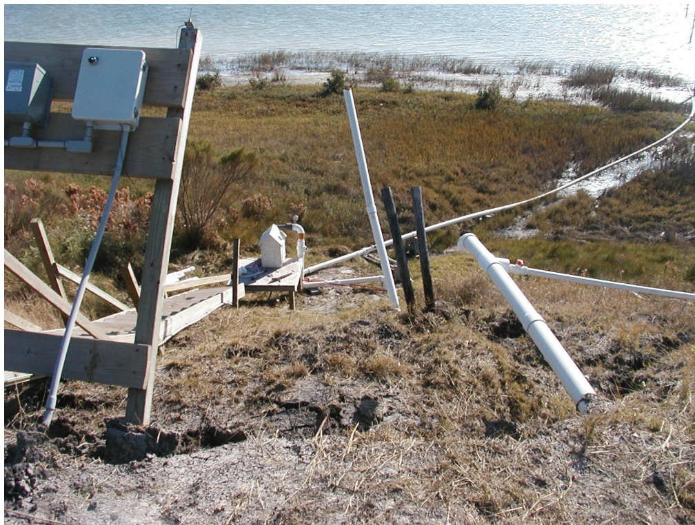
Figure 6.2. Photograph showing instability of hillside where intake pump is located after flooding.
