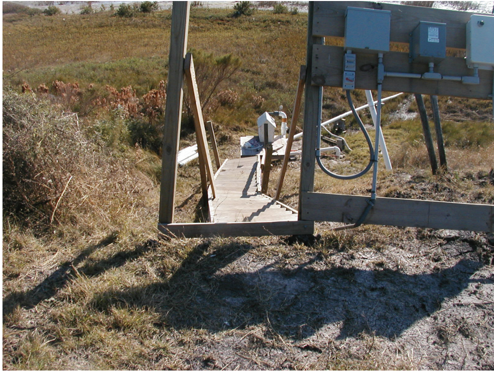
Figure 6.1. Damage sustained in December 2002 due to flooding at San Patricio.
