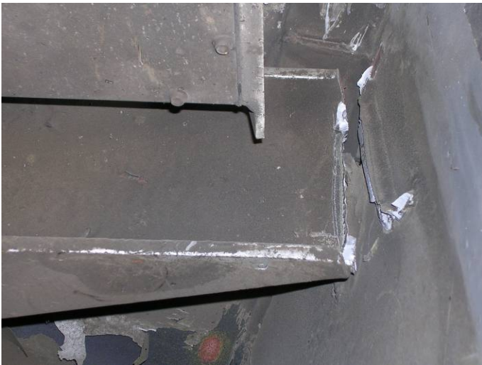
Figure 9. A Lateral Member Separates from the Draft Sill
