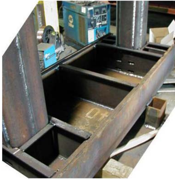
Figure 24. SOA End Frame in Fabrication; This is the End Beam Before the Top Plate was Welded on
