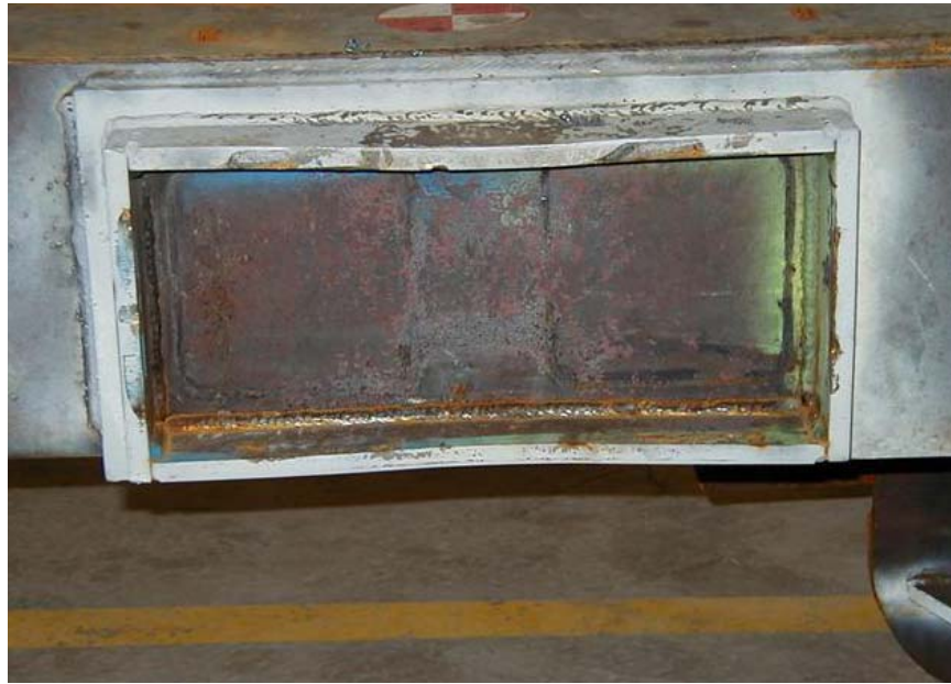
Figure 8. Back Surface of the End Beam After the CEM Test in the Area at Which the Primary Energy Absorber Contacts
