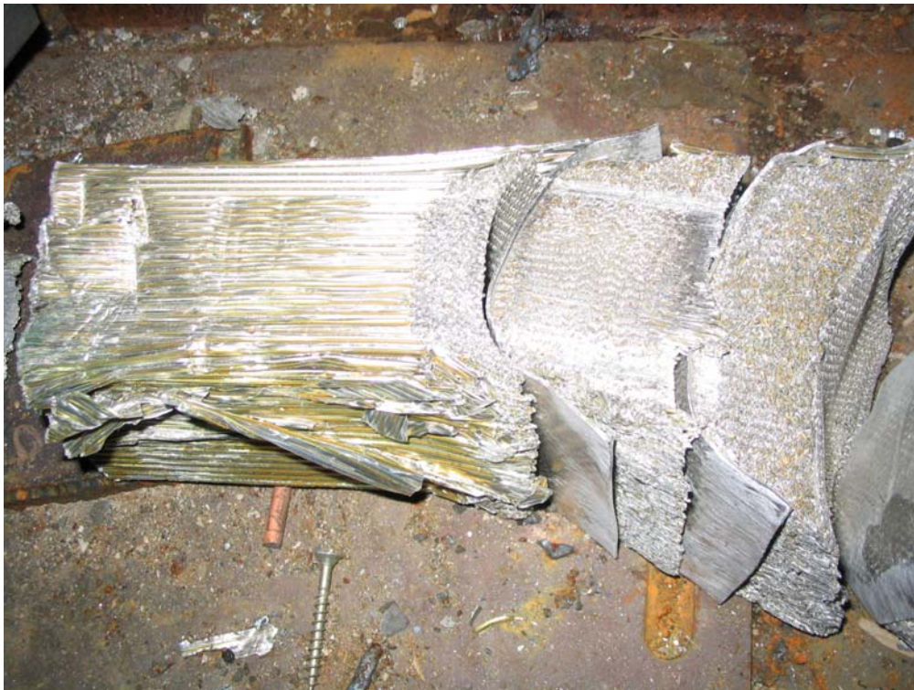
Figure 13. Roof Absorber Elements from End 248A That Experienced Substantial Crush
