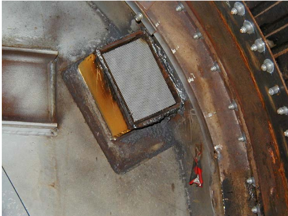
Figure 26. Inboard End of the Fixed Roof Absorber Tube After Removal of the End Plate to Extract Absorber Elements
