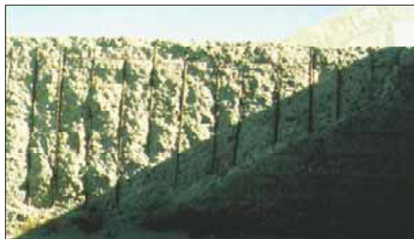
3.3. A spillway showing results of cyclic freezing and thawing.
