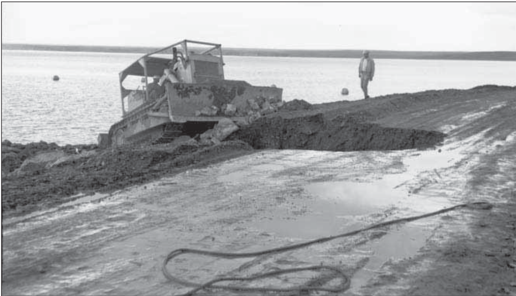
2.13. Fontenelle Dam: Crest sinkhole.
