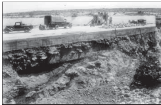
32.5. CCC men working on McMillan Spillway No. 2, Carlsbad Project, New Mexico, in 1938.
