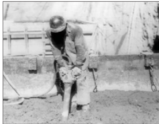
3.7. The use of vibrators allowed a lowered unit water content of the concrete mixture.
