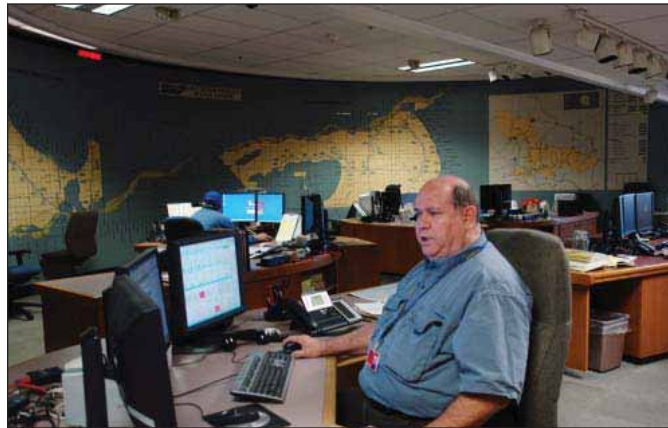
10.8. The Salt River Project's modern control room for its water system. Courtesy of the Salt River Project.
