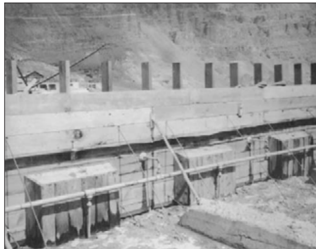
1.19. Owyhee Dam, Oregon. Grout pipes and shear keys on vertical contraction joint.
