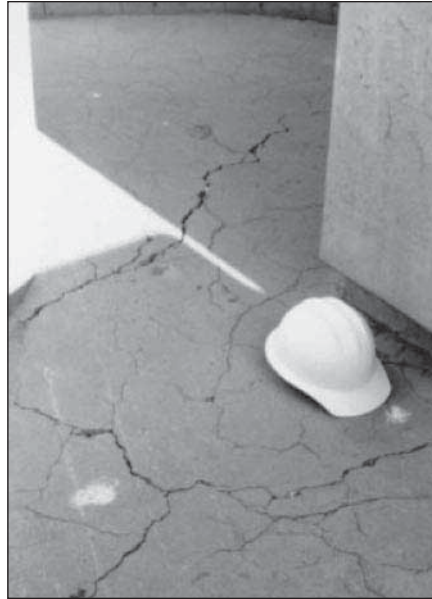
1.35. Cracking at Friant Dam due to Alkali-Aggregate Reaction, Friant Dam, California.
