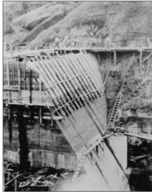
1.7. Construction at East Park Dam, California. Note the vertical formed contraction joint and concrete forms.
