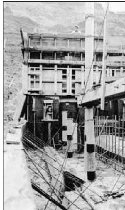
1.17. Owyhee Dam, Oregon. Tile formed drains, strain meter for Hoover test, and gallery reinforcement.
