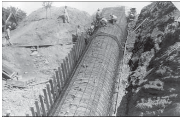
32.4. CCC forces placing steel reinforcement on the Stinkingwater Siphon, Belle Fourche Project, in 1938.
