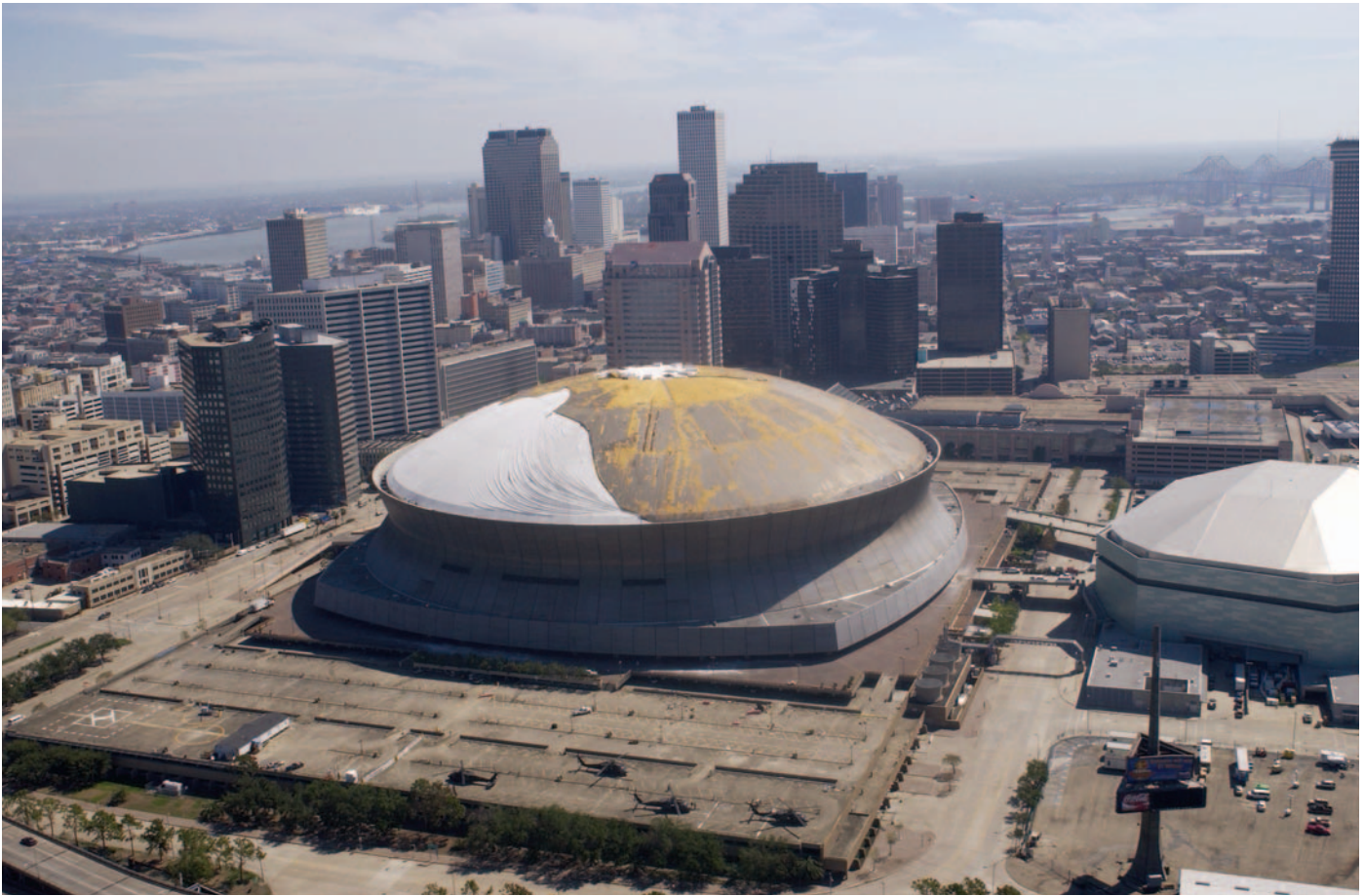
The Superdome with its storm-damaged roof U.S. Coast Guard photo
